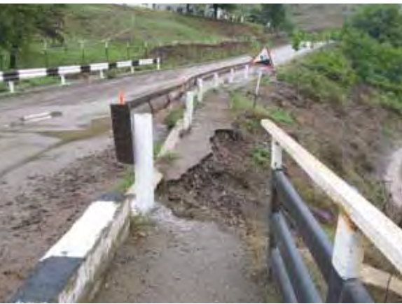
This road could not withstand a landslide and collapsed.
