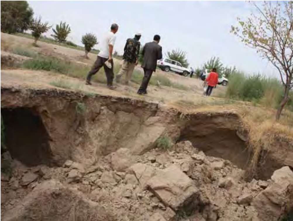
Land degradation led to the collapse of this road.
